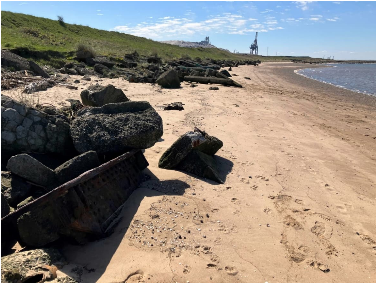
Plate 17A-12: View South-West Along The Edge Of Bran Sands, Showing Battered Edge Of Made Ground Underlying Redcar Bulk Terminal
